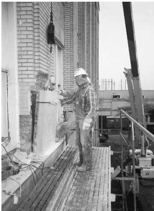
Mark Dietiker, Paul Misholek, and Jim Strong of Western Waterproofing spent three days separating and lowering the major decorative granite blocks from the front of the Lincoln Motor Company Administration Building.
