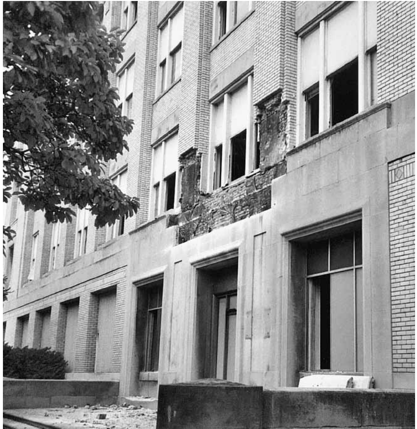
The front of the Lincoln Administration building after the surgery to save the decorative stone pieces. The building no longer exists, but it is hoped that the entrance will be reconstructed as part of a Lincoln vehicle display facility.
